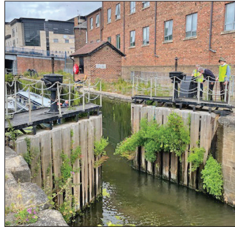
Gates showing poor condition
