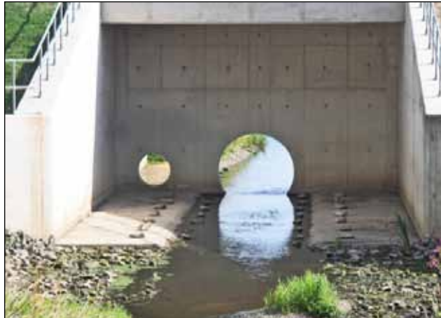
The dam before installation of the orifice plate. The smaller pipe is for emergency use and will normally be closed by a penstock. Photo by John Millett.
