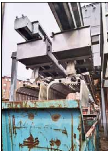
Mechanical grabs catch debris and remove it from stormy waters
