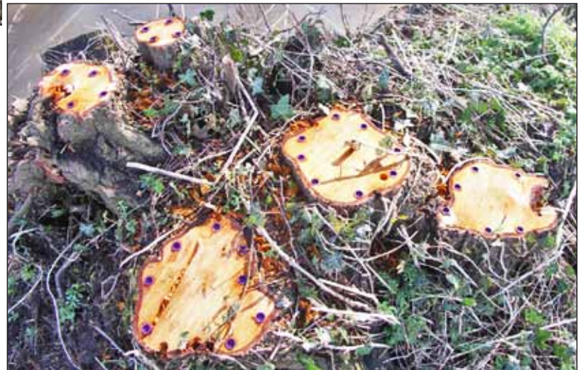
Top: The lock wall had been damaged by trees growing out of it for years
