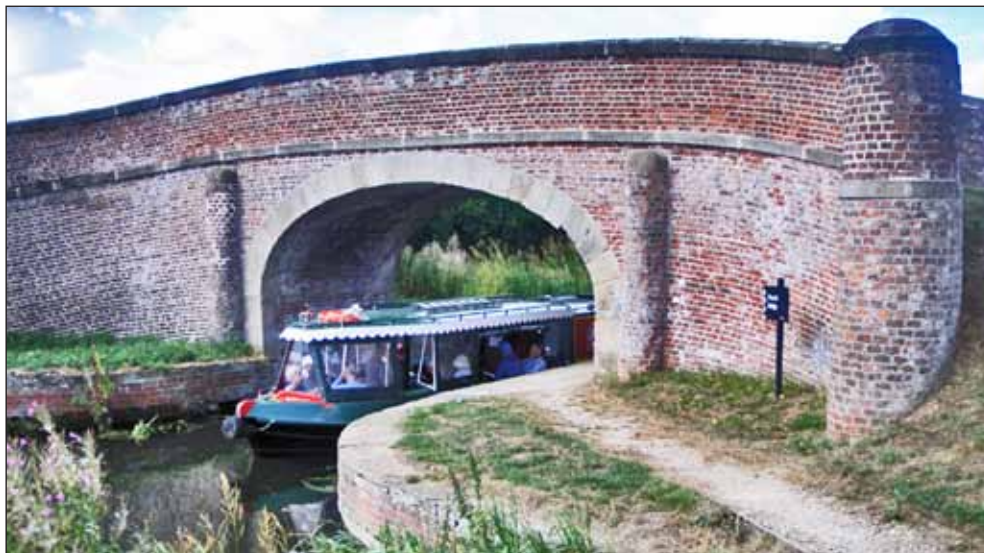
Church Bridge, Melbourne. Architecturally one of the best bridges on the canal system.
